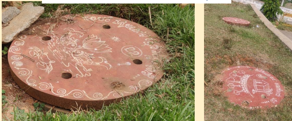
Photo 15: Percolation wells with clean visible tops
